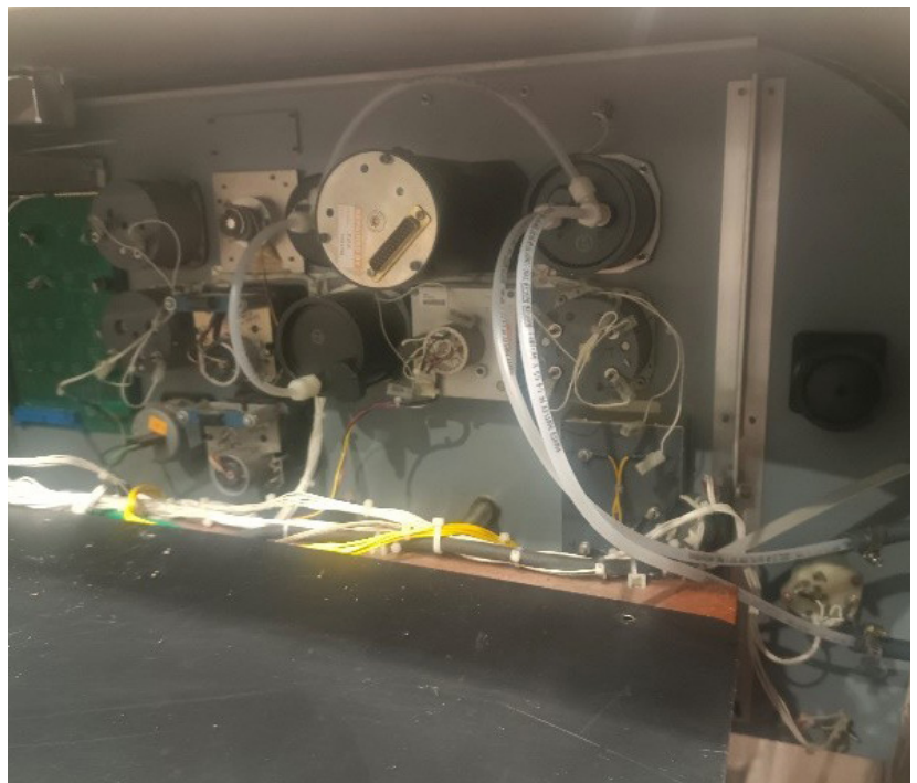
Figure 4 Pitot-static instruments installed and plumbed
